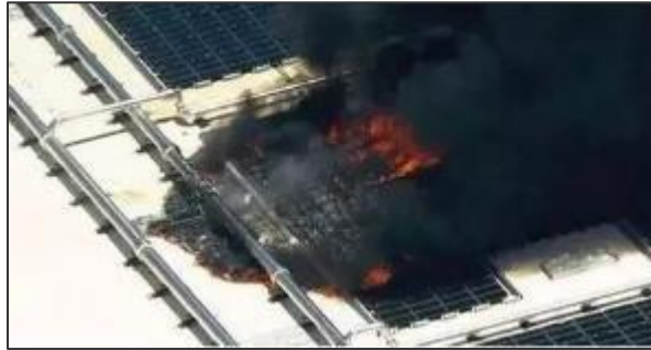
Apple Factory Photovoltaic Power Station Fire Scene Map
