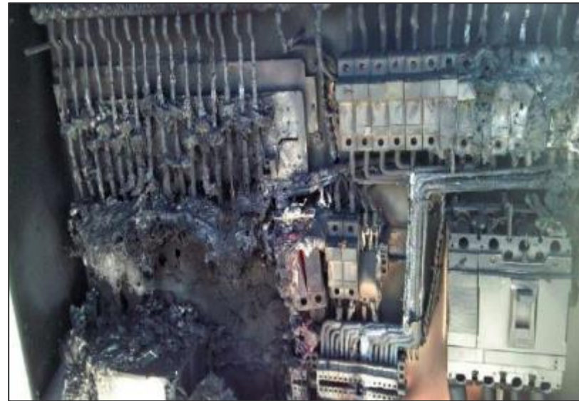
DC combiner box is burnt
