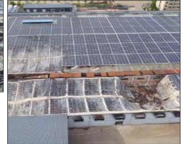
Fire scene map of roof power station in Zhejiang
